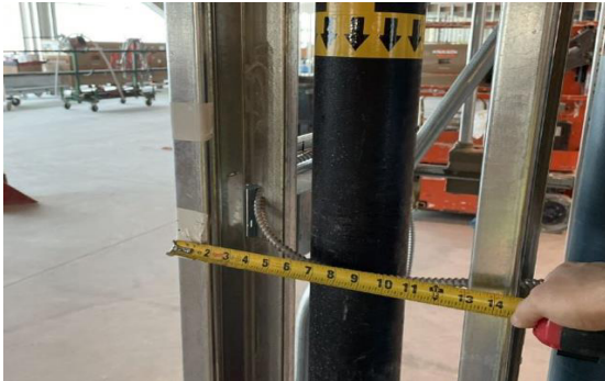
Figure 3: Photo Included in PDF Package Showing Pipe Location with Respect to Corner
