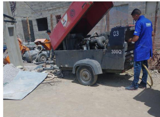
(b) evidence of breakage in the external plaster projection pump.
