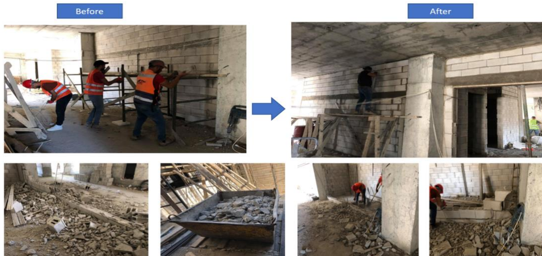
Figure 4: Lack of visualization for client review led to rework for a complete block wall
