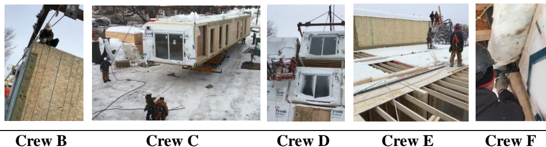
Figure 2: On-site pictures of crews B to F executing their specific tasks at study case A.
