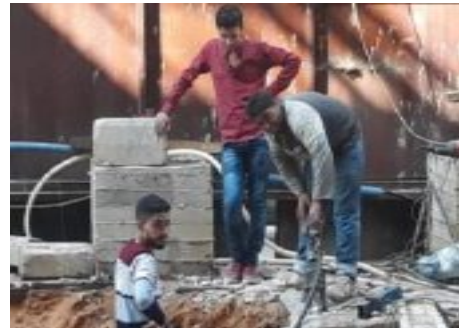
Figure 5- Workers not committed to PPE
