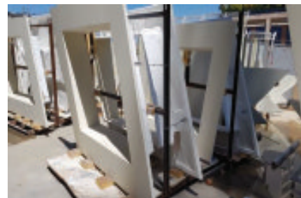
Figure 111: GRC Units Held on Rack
