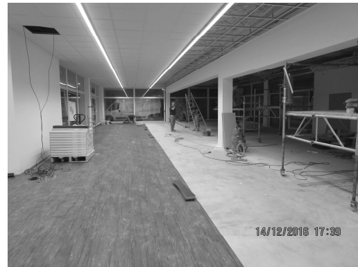
Figure 6: Takt Plan with Post-Its (left side) and impression of the construction site (right side)
