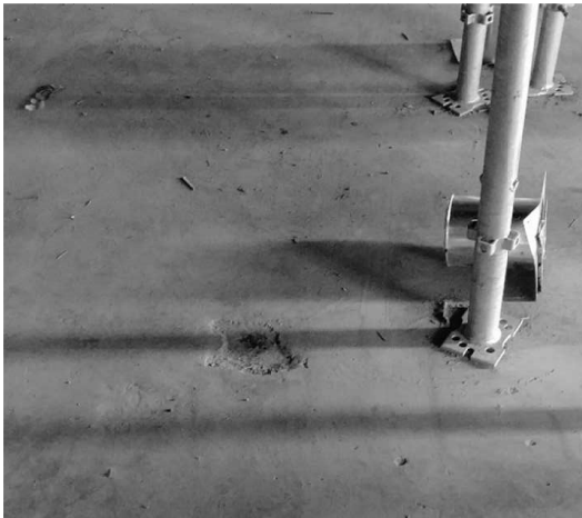
Figure 1: Floor concrete holes requiring patching work
