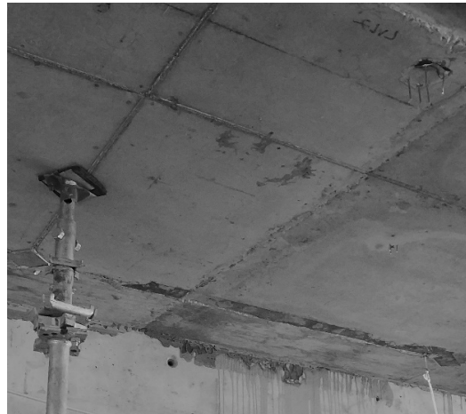
Figure 2: Ceiling and wall concrete finish requiring patching work
