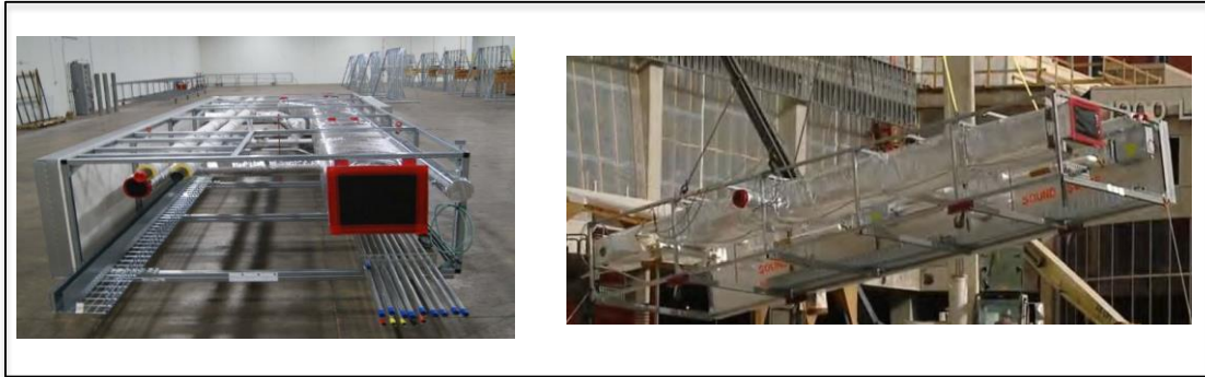
Figure 3: Example for prefabricated ceiling module stationary and installation at construction site (Figure p. 24 und 25 in N. U. 2013, USA)
